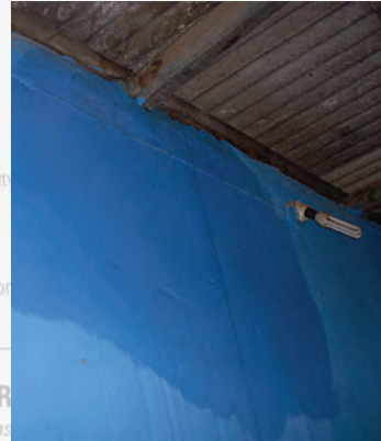
wet wall inside home [view from inside]
