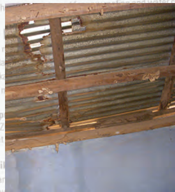
holes in roof [view from inside]
